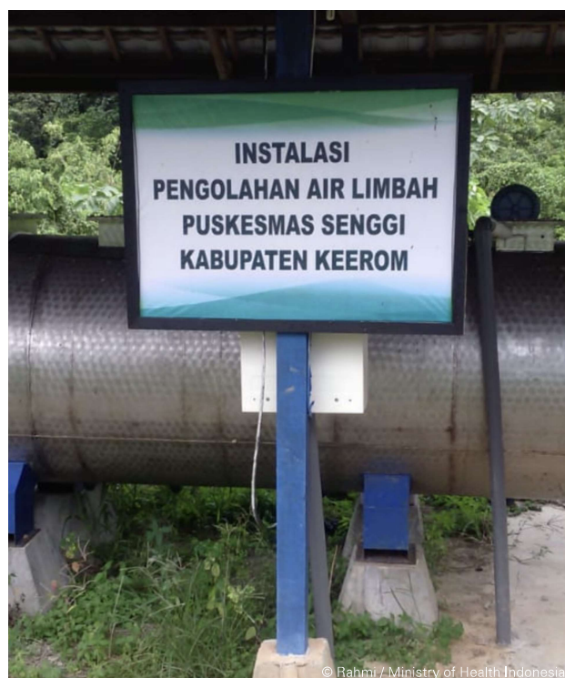
Wastewater treatment facility in Puskesmas in Keerom District, Papua
